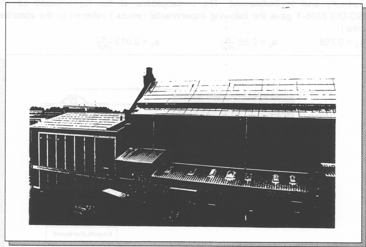
Figure B-3: Photograph of the cogeneration powerplant in Göttingen with the roof-integrated collectors on east and south array and the 'SolarWall' air collector (the third collector array is located on the other part of the flat south roof)
