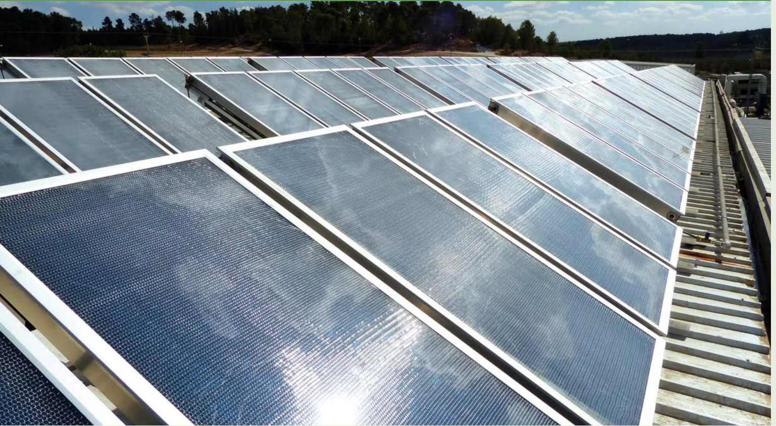
Flat plate collectors with transparent insulation used for a cleaning process in an Israeli dairy.
