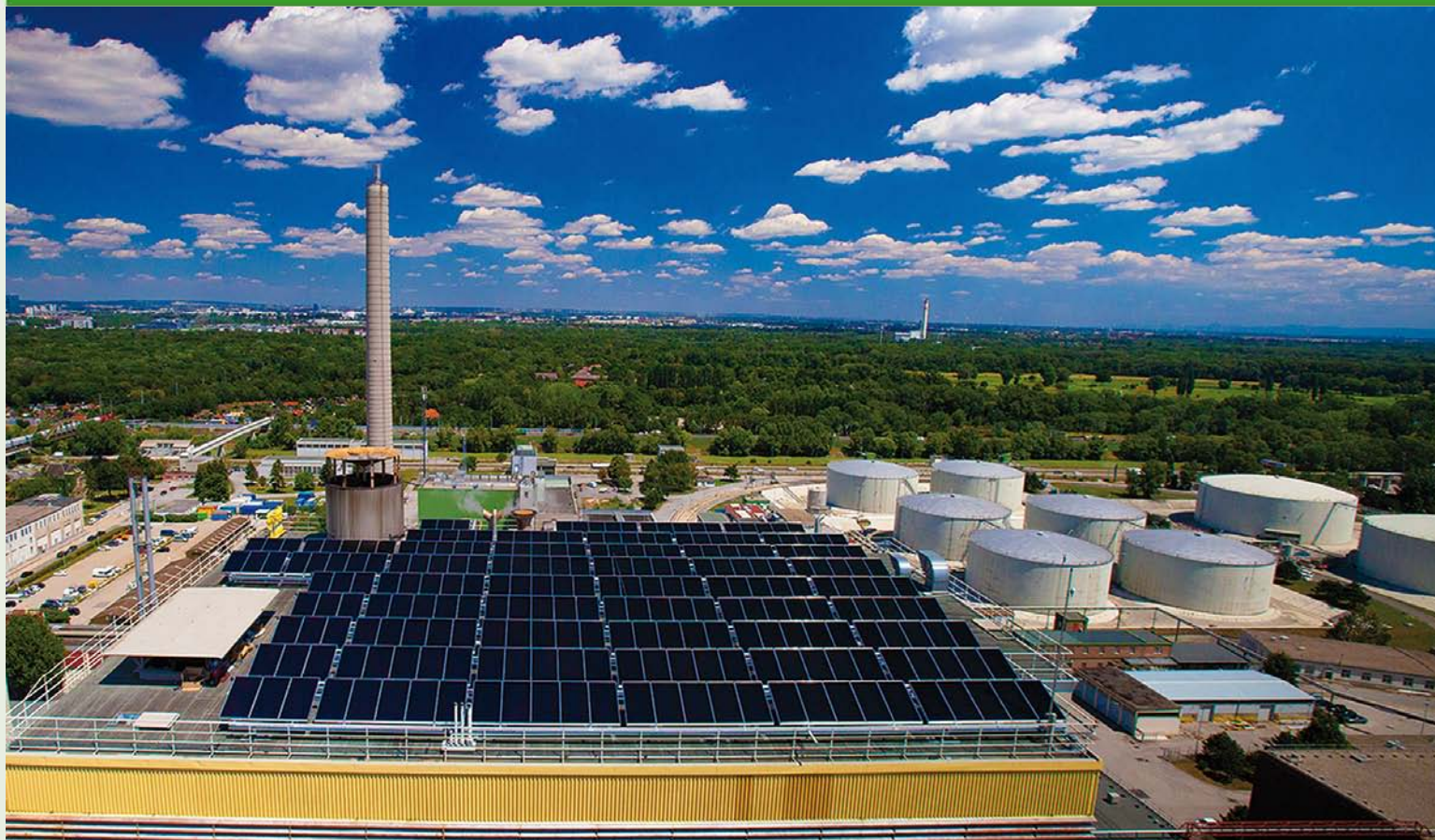
In Vienna 656 m 2 flat plate collectors were installed on the roof of a boiler house at a height of 70 meters. Photo: Greenonetec Solarindustrie GmbH
