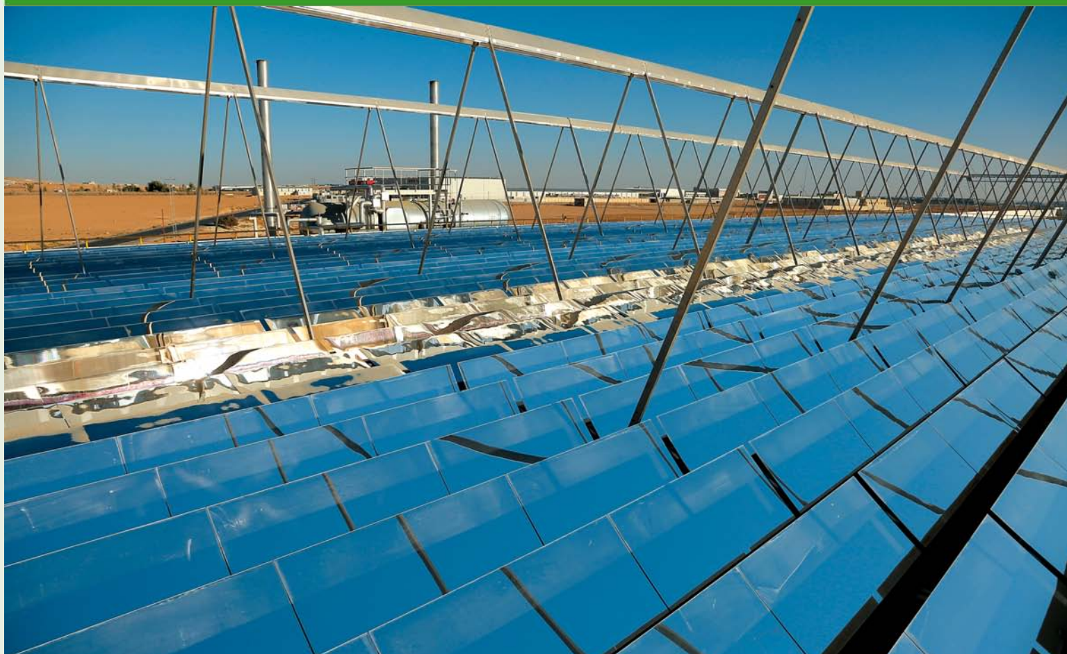
Linear Fresnel collectors used for direct steam generation for the solar cooling system at the Japan Tobacco International factory in Jordan.
