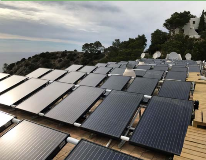
150 m 2 covered PVT collectors in Spain.
