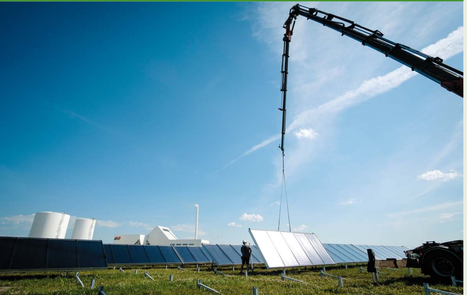
The Aabybro solar district heating system.
