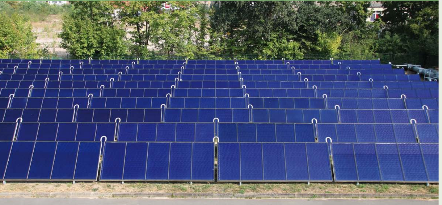
A 0.7 MW th solar thermal system supplies heat to the Berlin district heating network.
