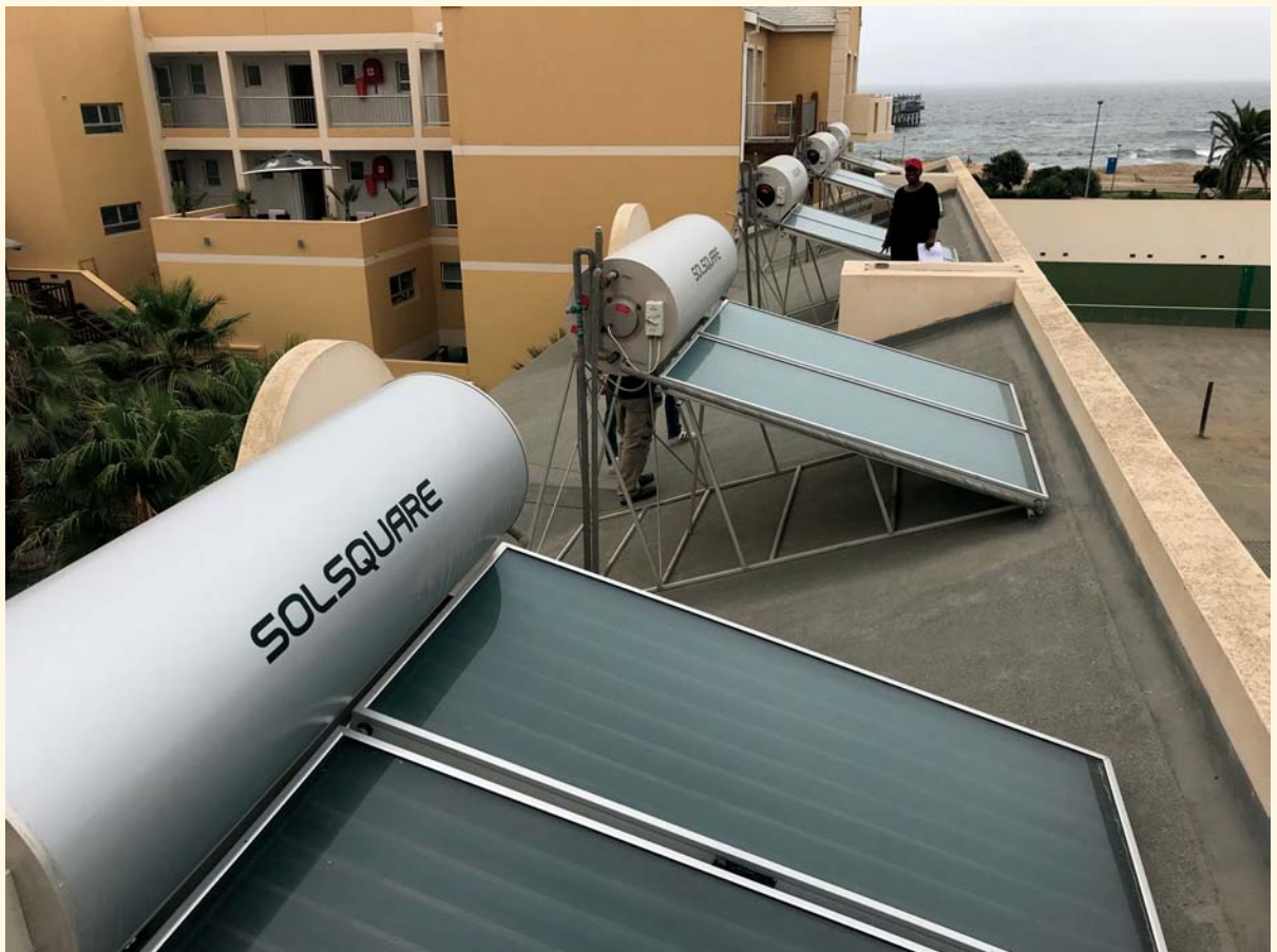
Thermosyphon systems at a hotel in Namibia.
