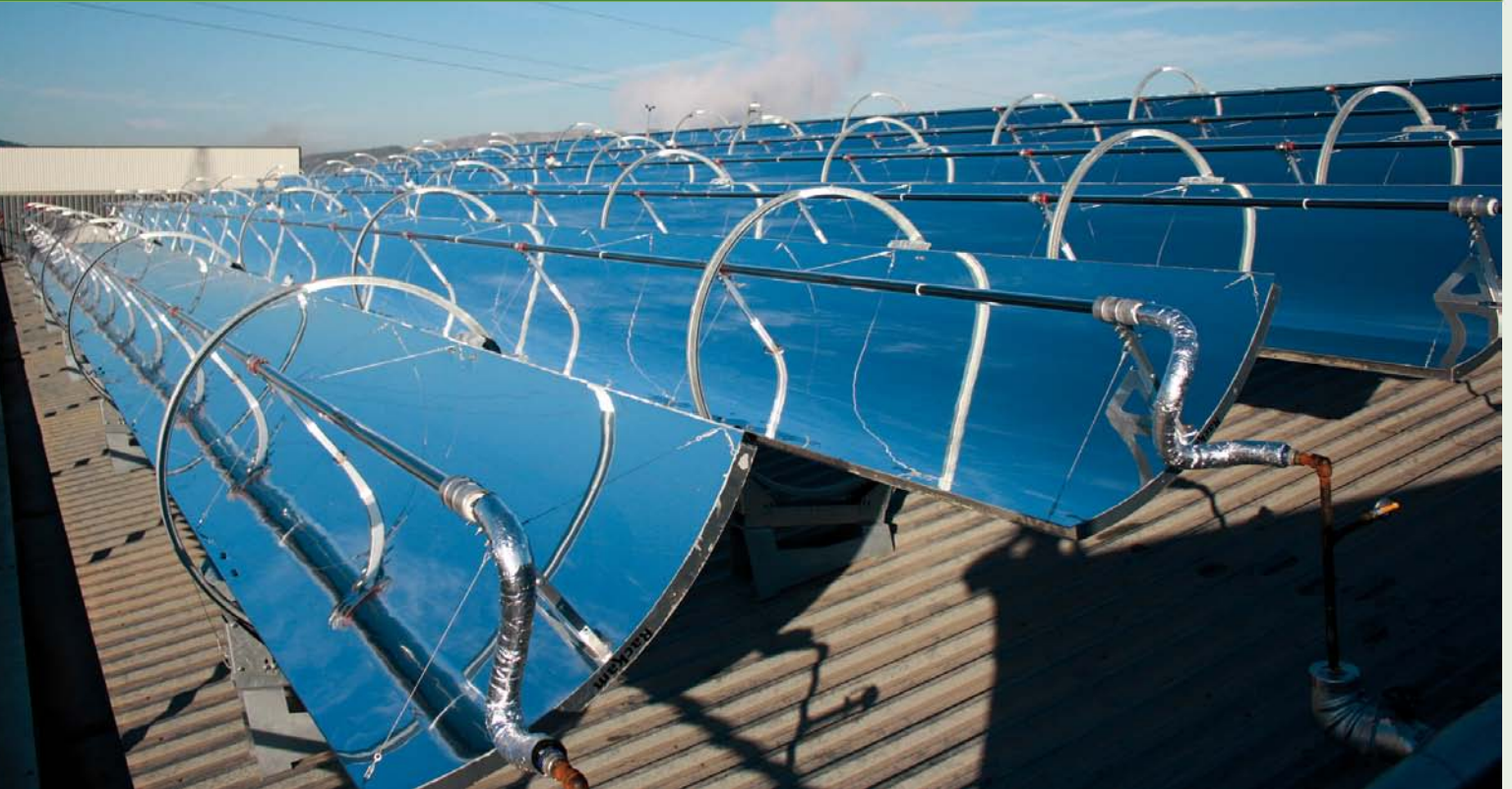
The food-processing plant of the company Papes Safor in Spain uses parabolic trough collectors.
