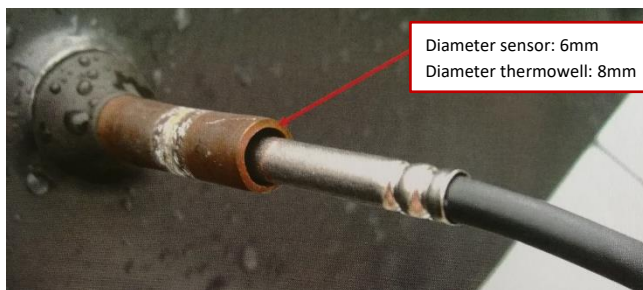
Figure 4: Air between sensor and thermowell due to incompatible diameters (Fischer, 2008).
